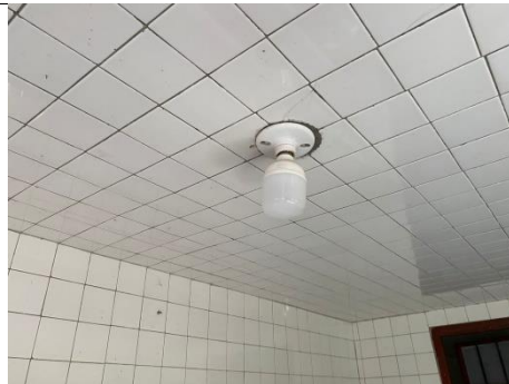
5. Luces led instaladas
